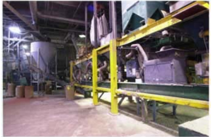
Because the loss-in-weight feeders were a proven success in Huntington, Ind., Isolatek also made the switch at its Stanhope, NJ., sift where the company manufactures wet spray-applied fire-resistive materials.
