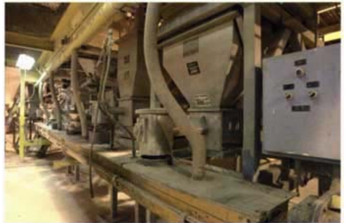
To improve process and quality control, Isolatek upgraded from volumetric to loss-in-weight feeders at its Huntington, Ind., site, where the company manufactures dry spray-applied fire-resistive materials.
