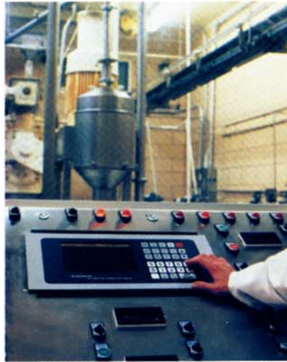
A controller oversees the entire batching and feeding system's operation, providing quick formula changes and variable production rates.
