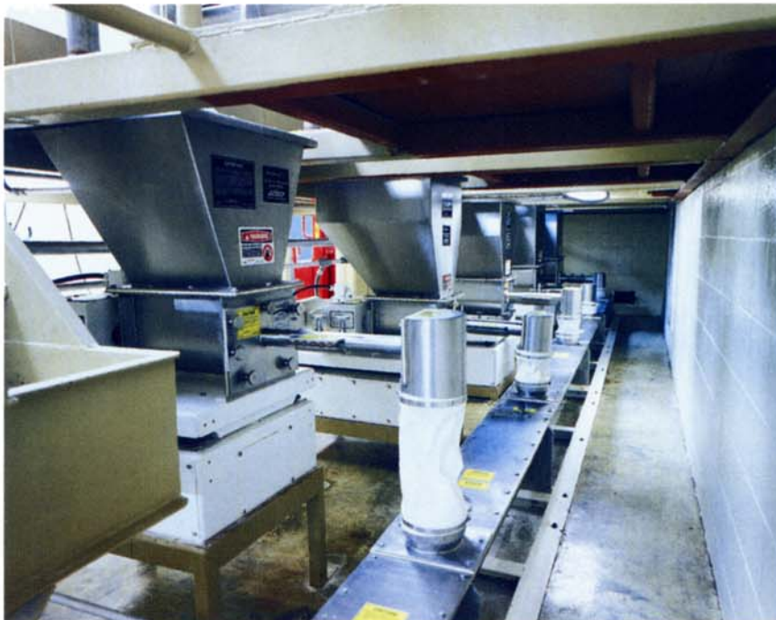
Loss-in-weight feeders meter the peanut butter ingredients to an auger preceding a blender that combines the ingredients before milling.
