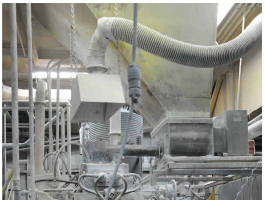
This volumetric feeder reliably meters a color concentrate into an extruder, ensuring batch consistency and continuous operation.
