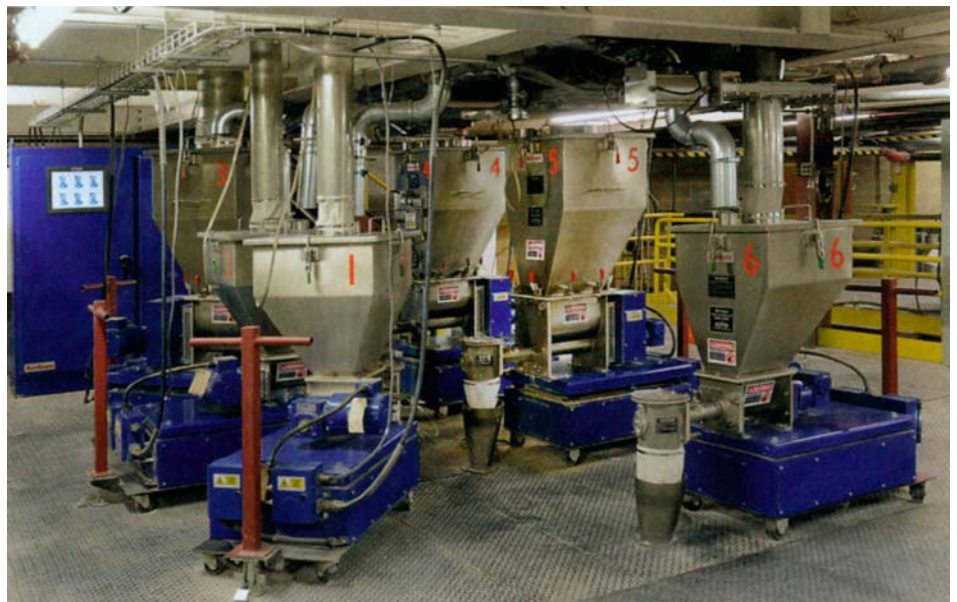
The six loss-in-weight gravimetric feeders and feeder control panel (back left) are installed on a mezzanine directly above the twin-screw extruder.
